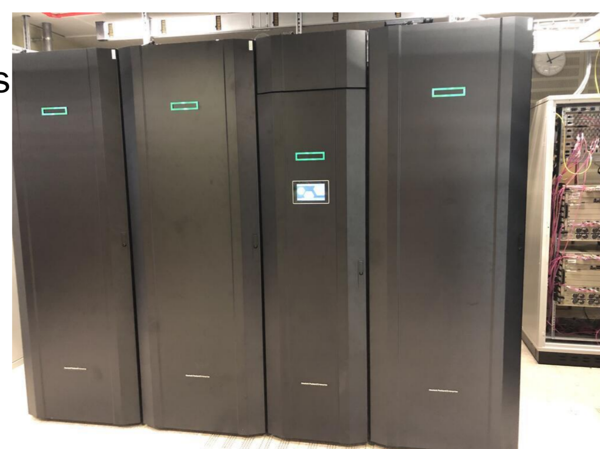
Figure 3: HPE-CRAY system at GeoSphere
